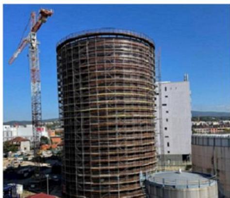
c) EL-TO Zagreb – Akumulator topline
