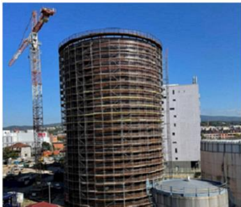
c) EL-TO Zagreb – Akumulator topline
