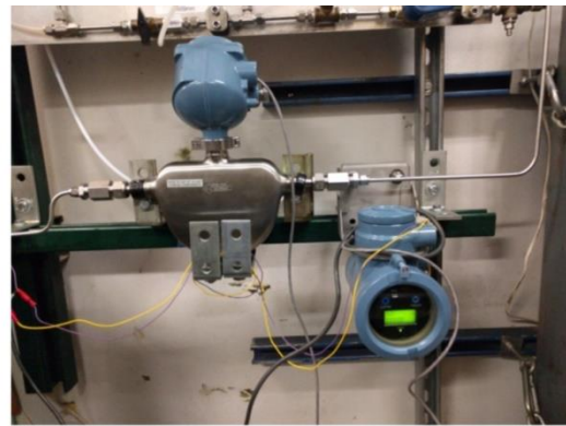
(b) METHANE FLOW METER
