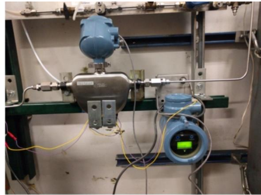
(b) METHANE FLOW METER
