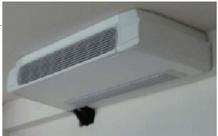
Ventilokonvektori: Fancoils SABIANA CRC 63 3,5 kW cooling (7/12 C) 4,13 heating (45/40 C)
