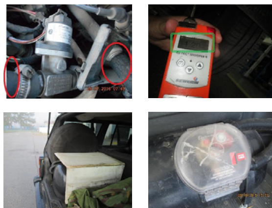
Figure 27: Cracked gas installation pipes and detected gas leakage (top). Inadequately protected gas tank (bottom left) and damaged gas tight housing (bottom right).
