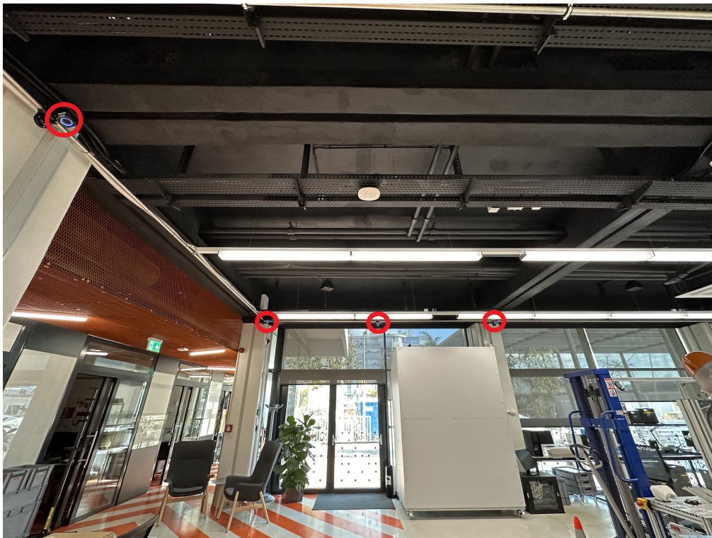
Figure 3.3: Camera setup view 1 (with cameras circled in red)
