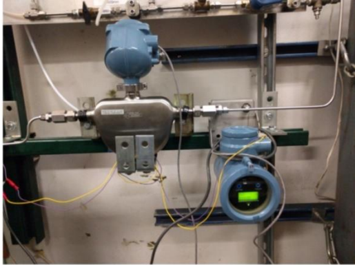
(b) METHANE FLOW METER
