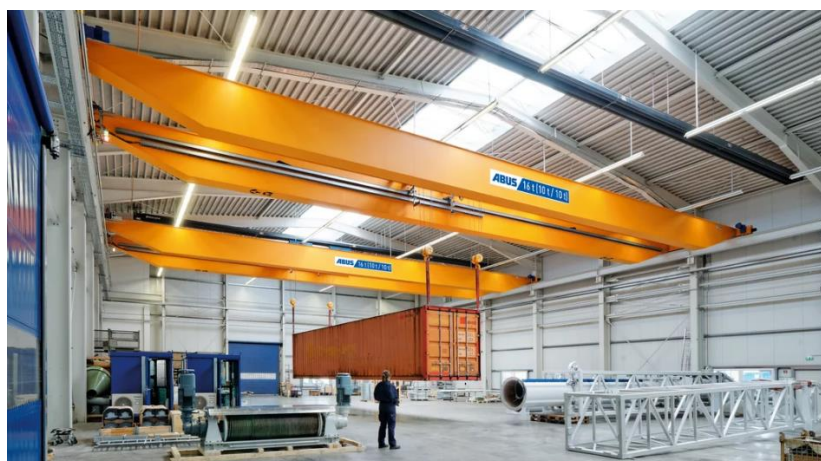
Slika 4. Abus crane system – Double girder overhead travelling crane
