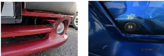
Figure 18: Cracked front bumper (left) and a roof spoiler improperly mounted by rear window drilling (right).
